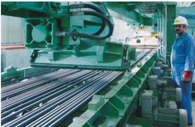
Steel plant motors – transport material for coiling
